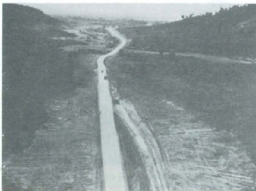
LAND CLEARING ON BOTH SIDES OF A PUBLIC ROAD to reduce chances of enemy ambush.
