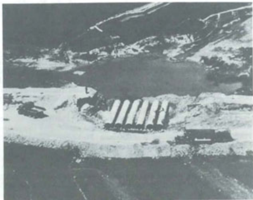
EARTH-FILL BYPASS FOR BRIDGE DESTROYED BY ENEMY. Six-barrel culvert will replace bridge.
