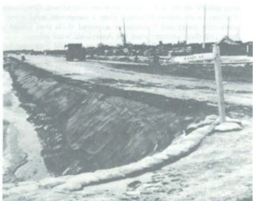
EROSION CONTROL AT DONG TAM in the delta where sandbags and burlap treated with penepime (asphalt derivative) were used.
