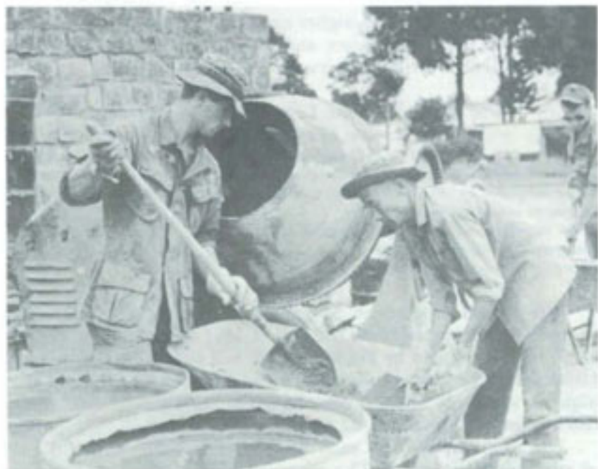
VIETNAMESE BUILD A MASONRY GATE AT BAO LOC for the agriculture school with the aid of the 116th Engineer Battalion.
