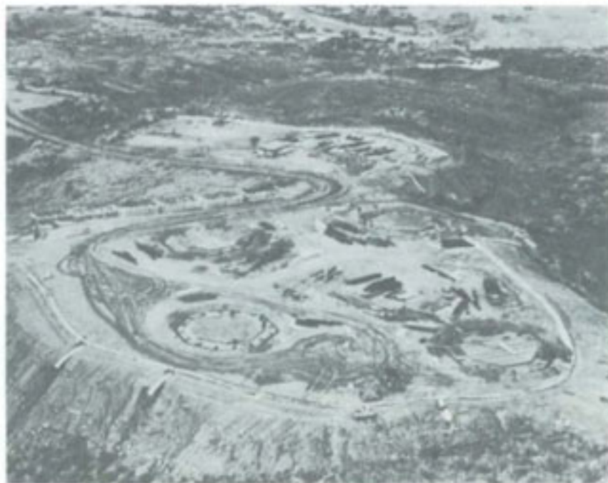
ARTILLERY FIRE SUPPORT BASE known as Landing Zone Uplift under construction by 35th Engineer Battalion.
