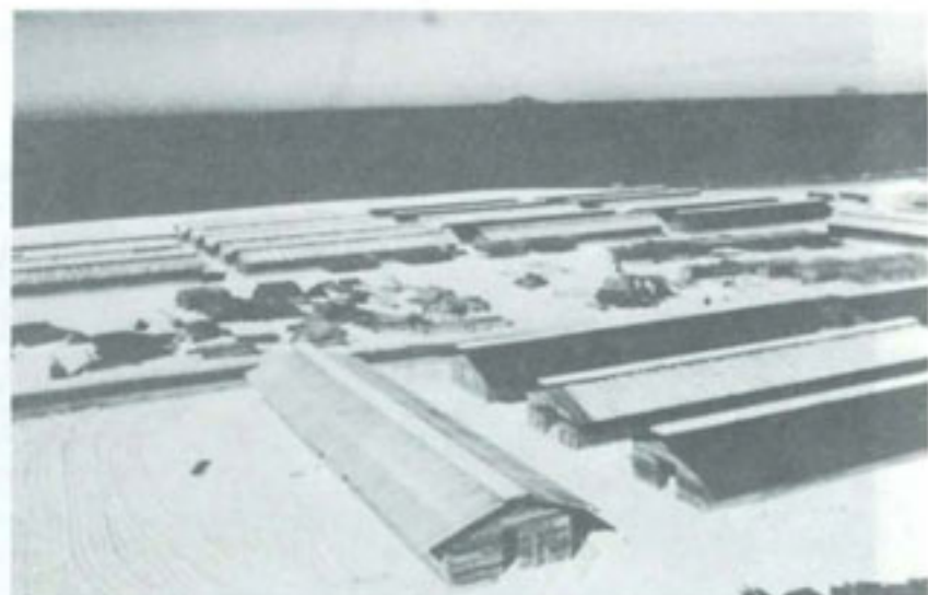
CONVALESCENT HOSPITAL UNDER CONSTRUCTION AT CAM RANH. Buildings are made of frame sections, precut and prefabricated on site, and have concrete floors and sheet metal roofs.
