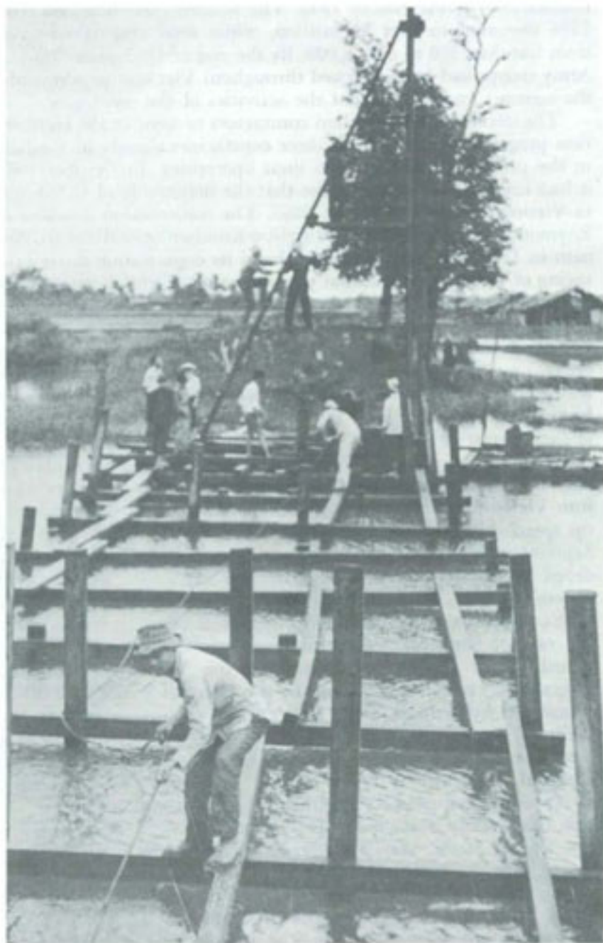
VIETNAMESE VILLAGERS BUILDING A BRIDGE. U.S. Army provided materials, equipment, and technical aid.
